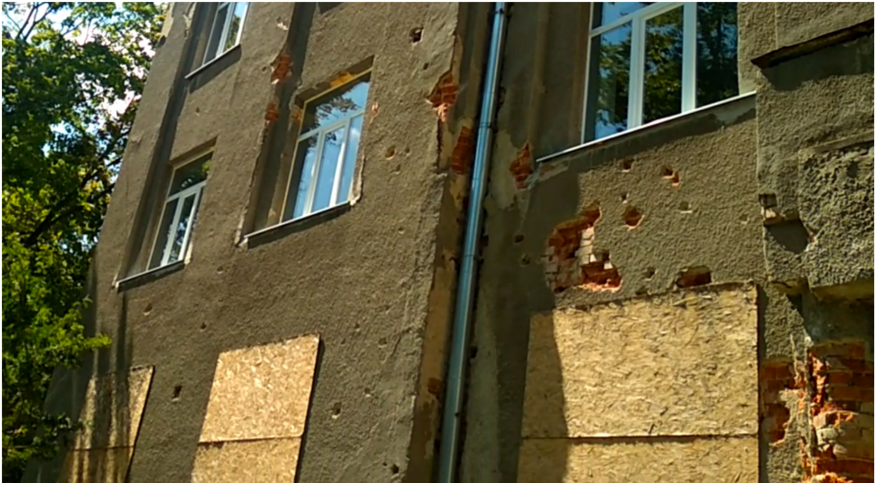
Damaged "Slovo" Building
