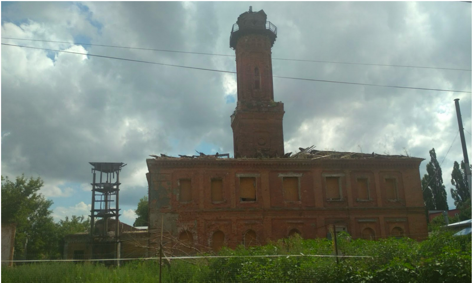
Damaged firefighter station in Kharkiv. This station was monitored by our team first time in march 2022 see chapter 3.2.Damages repairs in long term perspective
